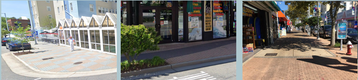
Existing pavers are dated and inconsistent. Some are no longer stocked and difficult to match when replacements are needed. Settling has created uneven surfaces and ADA issues.
