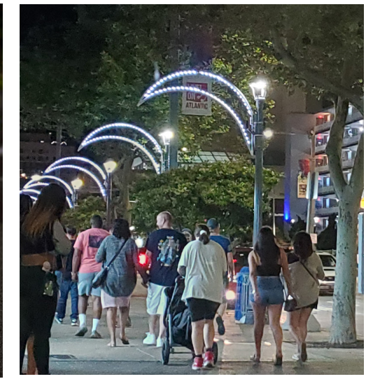
Accent Light Elements Attached to Street Light Poles
